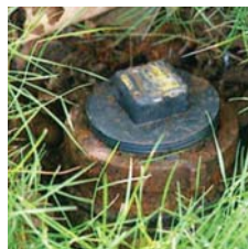
Cleanout sanitary sewer line access
